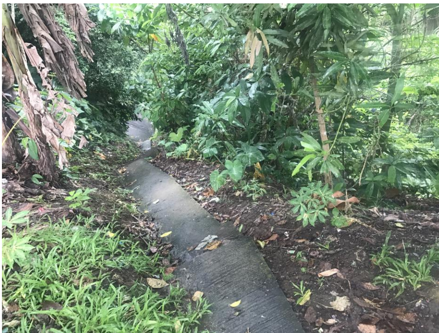
Figure 4. Picture taken during the actual visit of the CDRA Core Team to inspect damages on pathways
