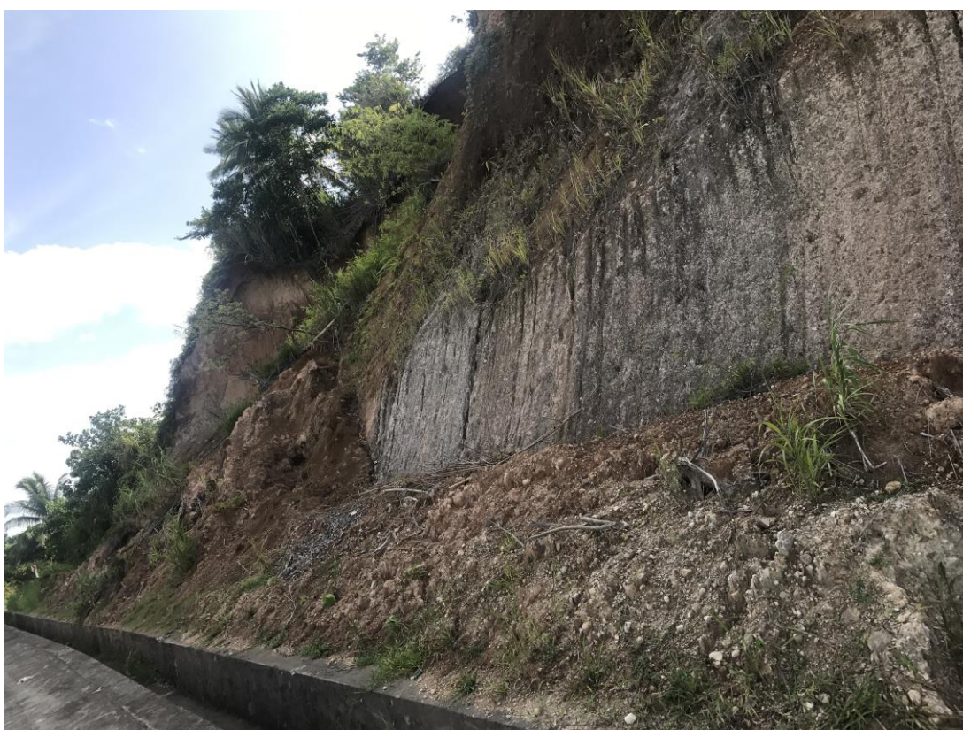
Figure 92. Landslide-prone area along the road in Barangay Naagtan.
